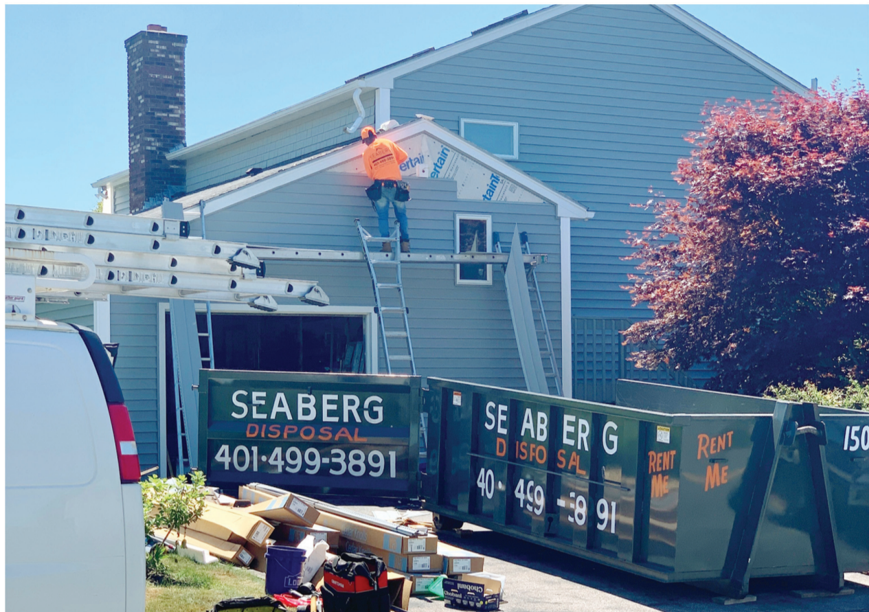
The dependable crews of Seaberg Construction are laboring to get your home improvement project, just like this siding job, finished in a timely manner – no short cuts, just good old-fashioned hard work.
